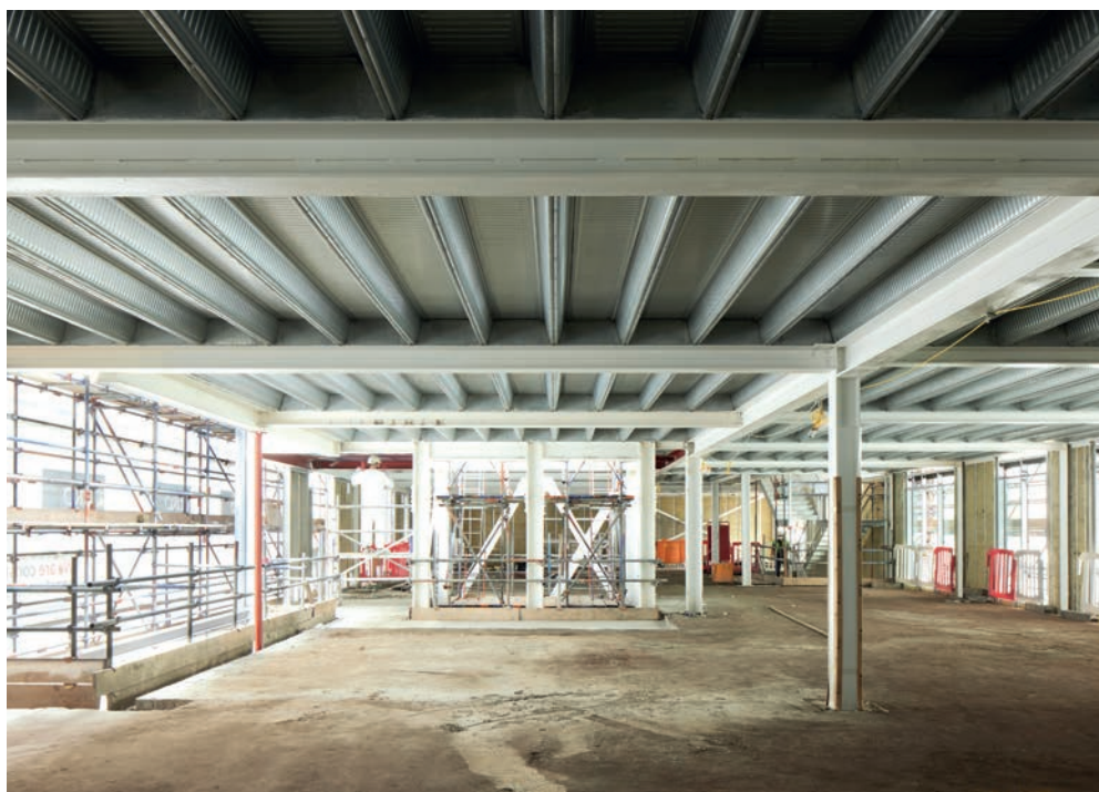
FIGURE 5: New composite floor for one of additional storeys, and view of central lift core
